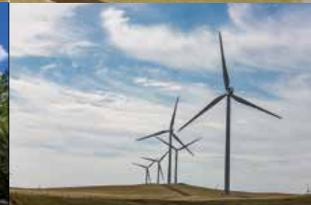
▲ Stantec paleontologists helped excavate 17 turbine foundations for the Blackspring Ridge Wind Power Project in Alberta, turning up dinosaur bones, plant fossils and microfossil sites in shellbeds that contained small bones, teeth and scales from dinosaurs, turtles, crocodiles and fish. The fossils are now at the Royal Tyrrell Museum of Paleontology in Drumheller
