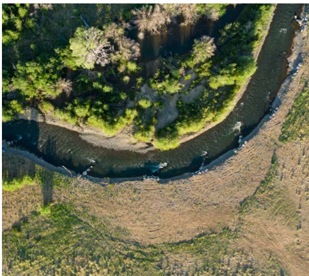
Figure 1. Natural restoration work on the Alamosa River included installing hydraulic structures to better manage erosion and sediment deposition.
